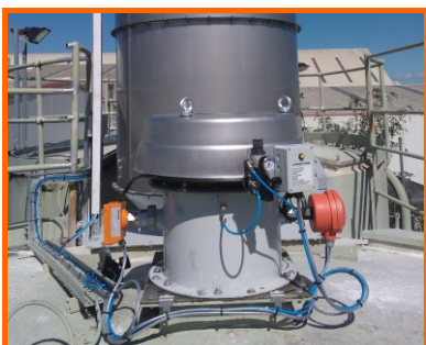
Latest testable silo instruments
