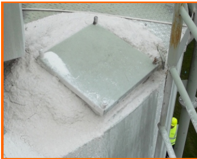
Product discharge from the PRV
