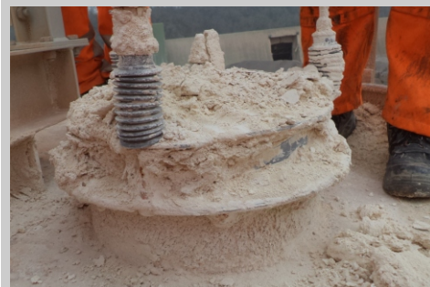
Pressure relief valves (PRV) are the last line of defence against over-pressure. With effective protection and servicing, blocks like the example above can be avoided.
