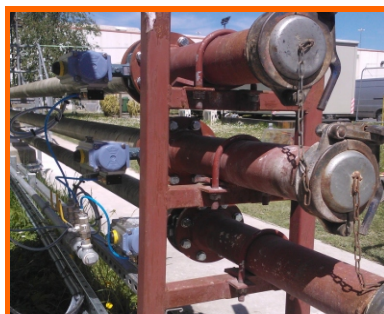
Valves fitted for auto shut-off
