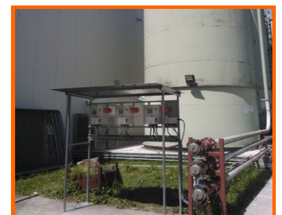
Display and control at fill point
