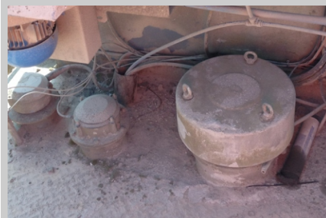
After physical testing, this PRV and pressure sensor failed to operate at the correct set points. Previously this was serviced with only a visual inspection!
