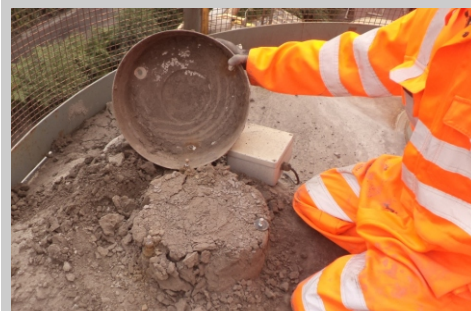
This PRV appeared fine, but an inspection under the lid reveals the opposite. This problem would indicate the silo safety system has totally failed!
