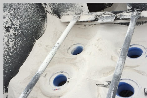
Damaged and neglected filter cartridges will cause emission issues if they burst, or if they are completely blocked they have the potential to cause serious silo damage!
